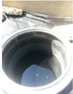
Excessively high water table
